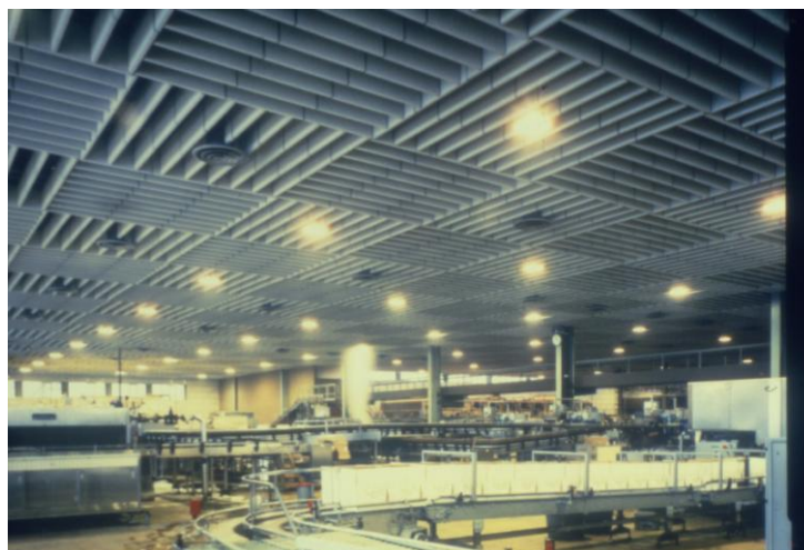
Figure 1 Sound absorbing baffles in a bottling plant
