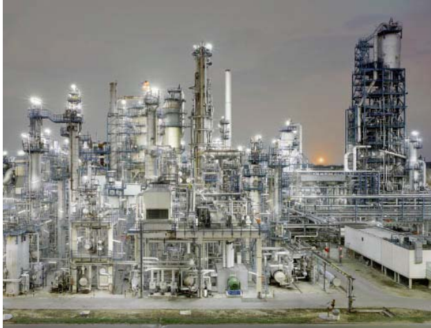
Figure 8 - Acoustically semi-transparent structures in a refinery.
