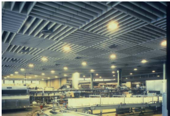
Figure 1 Sound absorbing baffles in a bottling plant
